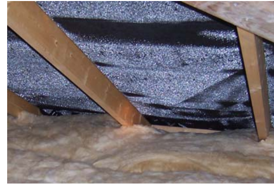
Photograph shows how condensation can form on the underside of an underlay during the drying out period
