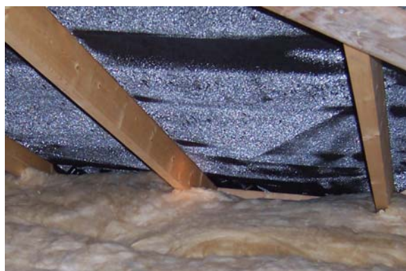
Impermeable (Type HR) underlay with flocked underside showing condensate being held
