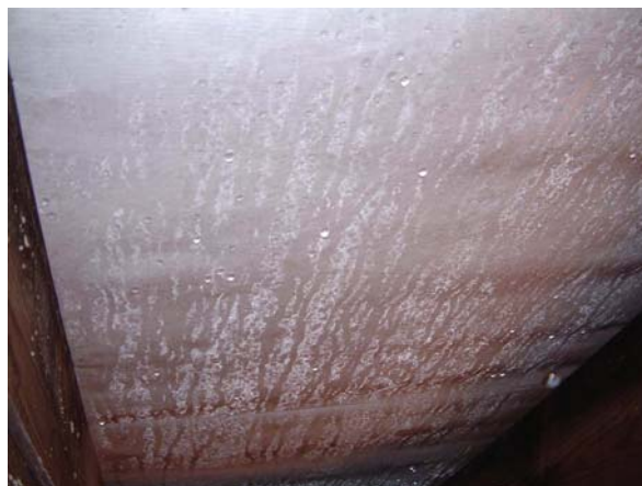
Vapour permeable underlay (Type LR) with smooth underside showing condensate run off and dripping
